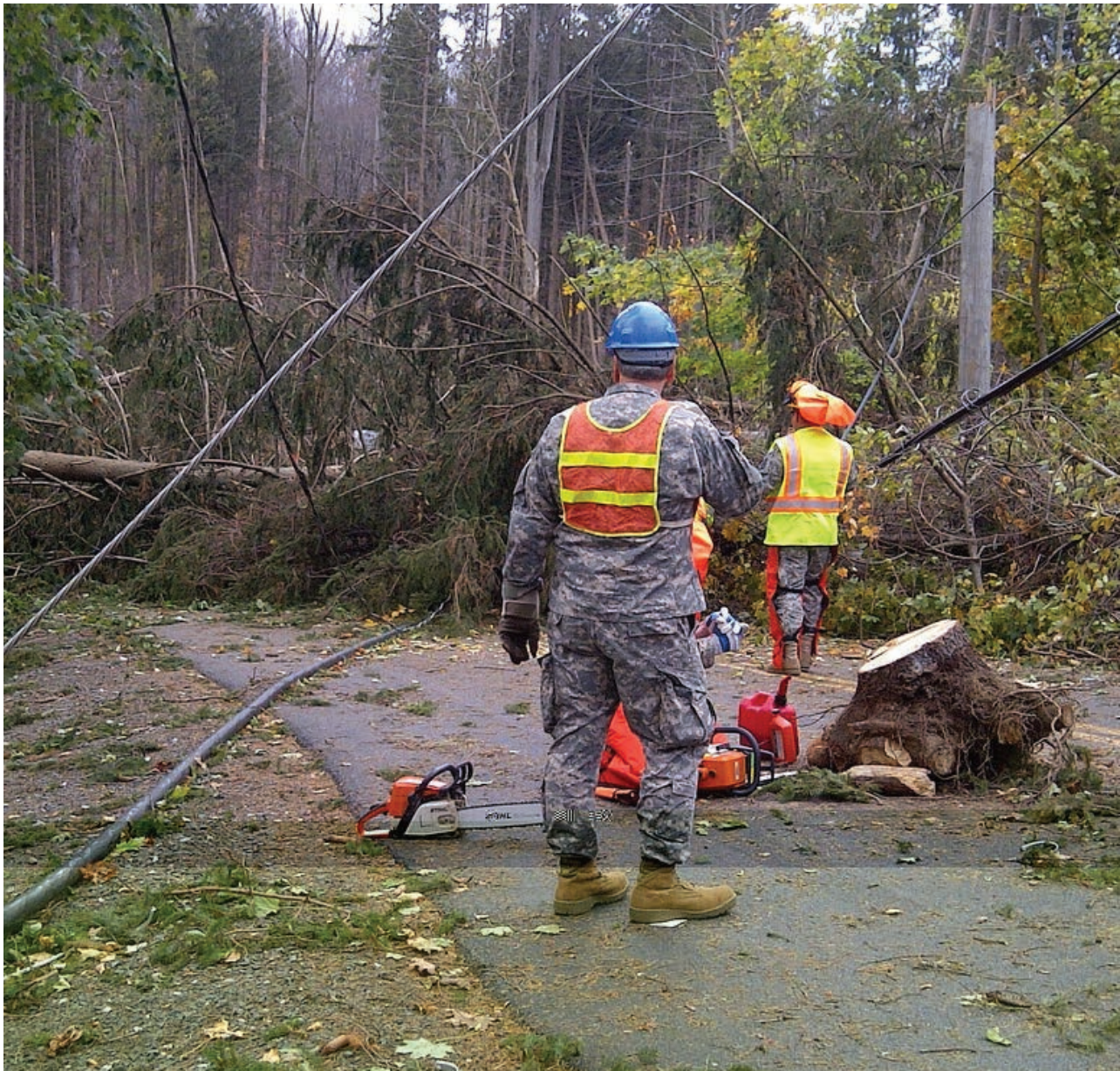
National Guard clearing trees and debris from roadways in Bedford, NY, after Superstorm Sandy.
