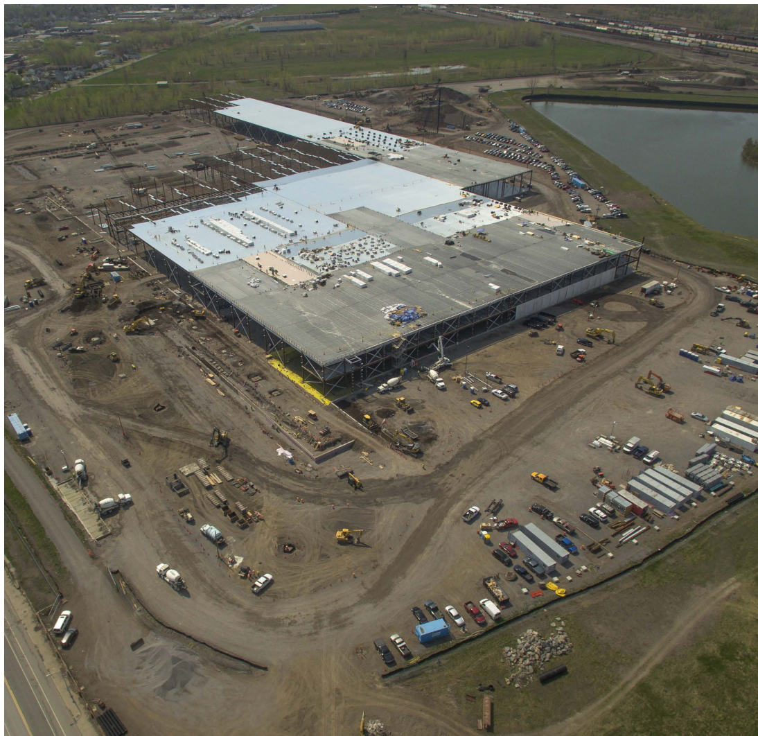
Aerial view of the future 1.2 million square-foot SolarCity Giga Factory in Buffalo, NY.
